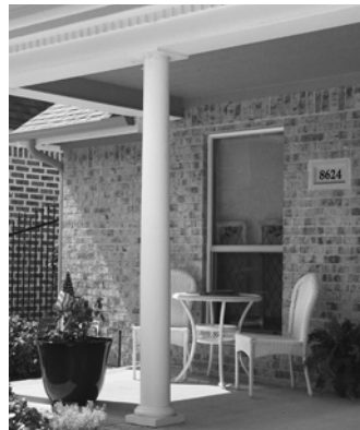
Window lacks muntins.
