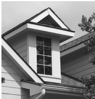
Dormer overhang is too deep.
