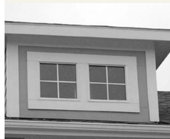
Overhang is too deep, too much wall area, trim width is not proportional to window size.
