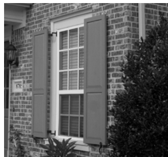
Surround and lack of brick mould make this window inappropriate.
