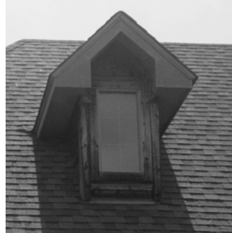
Overhang and rakes are too deep.
