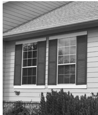
Header and sill are too wide.
